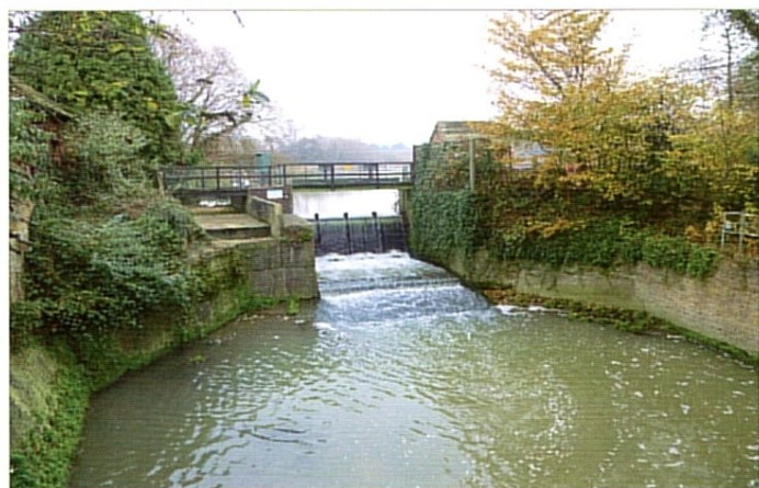
The problem sluice at Warnham Mill. Picture - Nigel Harris
